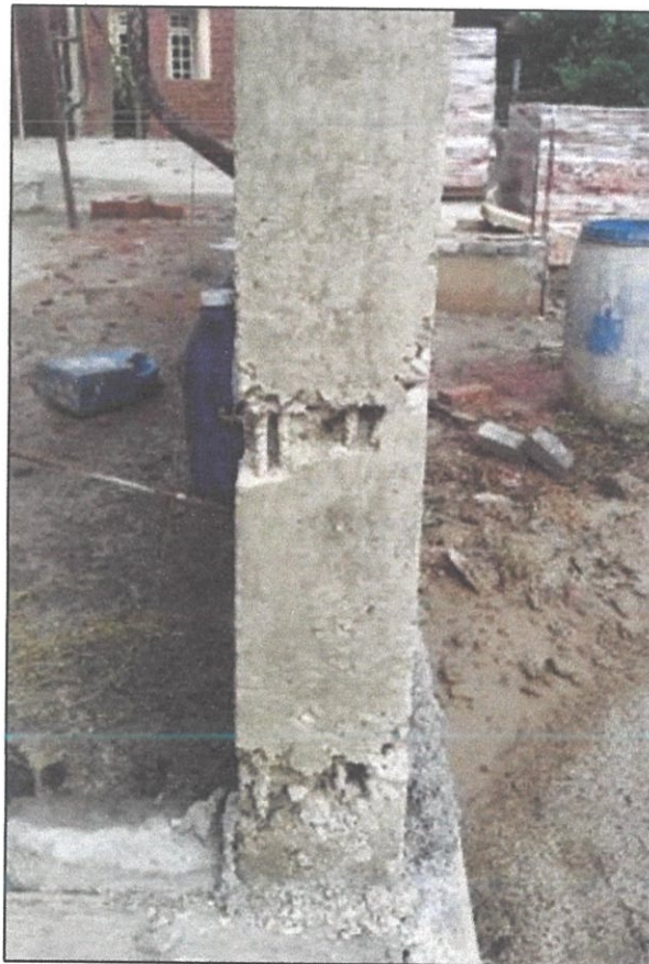
Figure 3.19: Honeycomb on Column
