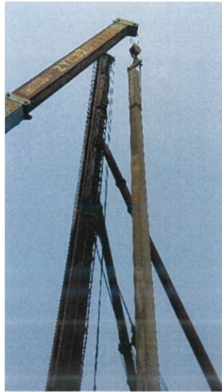
Figure 3.6 show the pile will lifted by crane and pile should be put into the grip of the jack in machine and operator will gripped the pile body.
