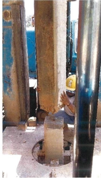
Figure 3.9 show the 6m pile attached with the 12m pile for the extension work.
