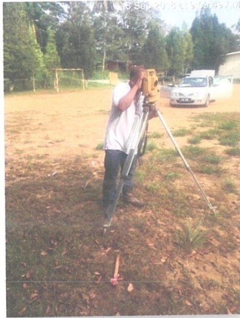
Photo 3.5 Land Survey come to calculate and set up the perimeter of the area.
