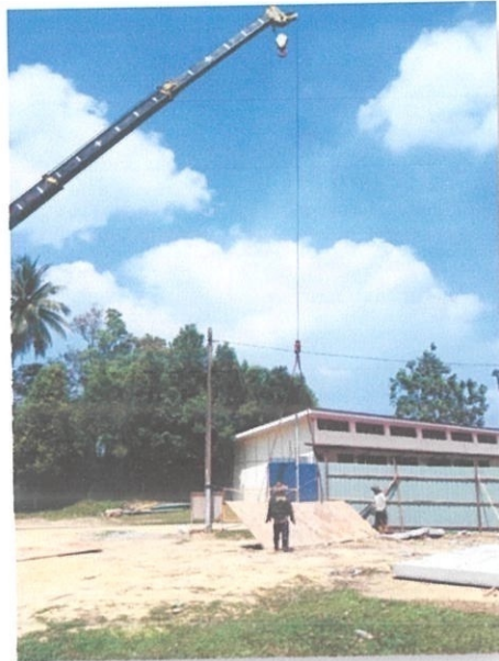
Photo 3.15 The Crane is used to lift up a platform for lorry going through.
