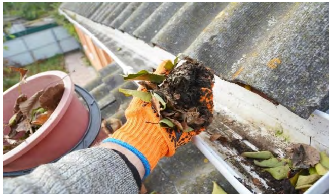
Figure 2: Dried leaves Clogged in the Gutter
